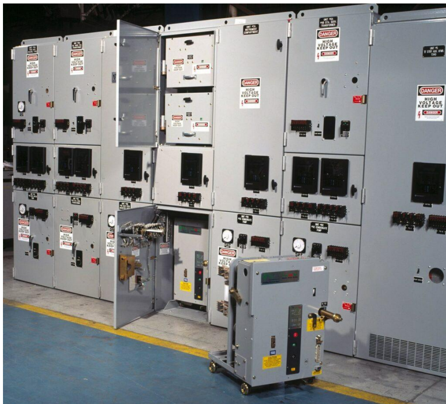
Photo of MV switchgear lineup from a PCTX project
